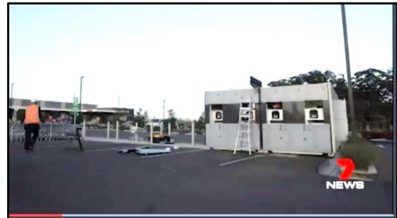
The first on site installation at Spring Farm's Woolworths Supermarket in Camden, NSW 16 th of October
